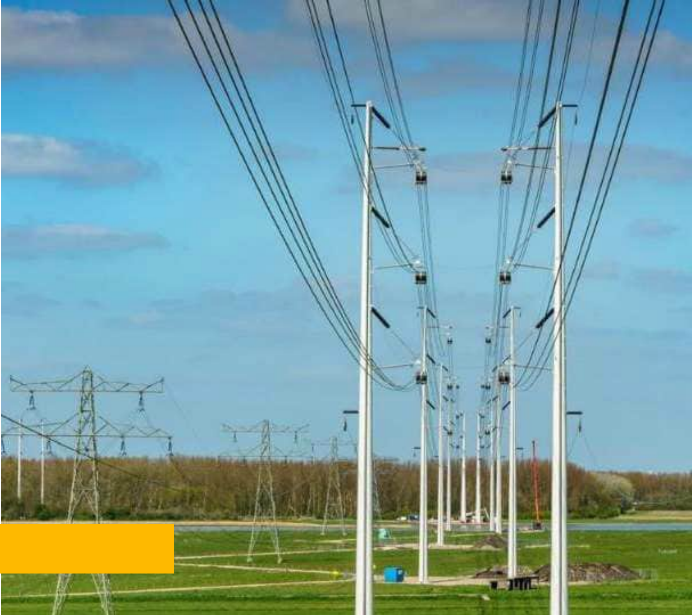
WINTRACK II - TENNET INFRA
