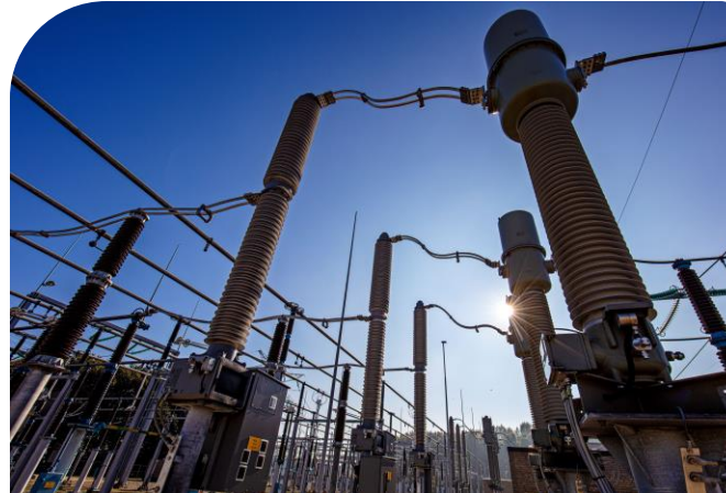
EU-303 high-voltage substations for TenneT
