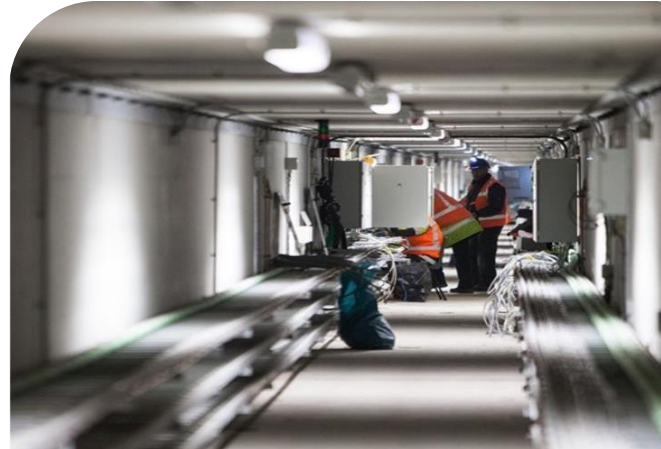
Maintenance and operations of technical installations
